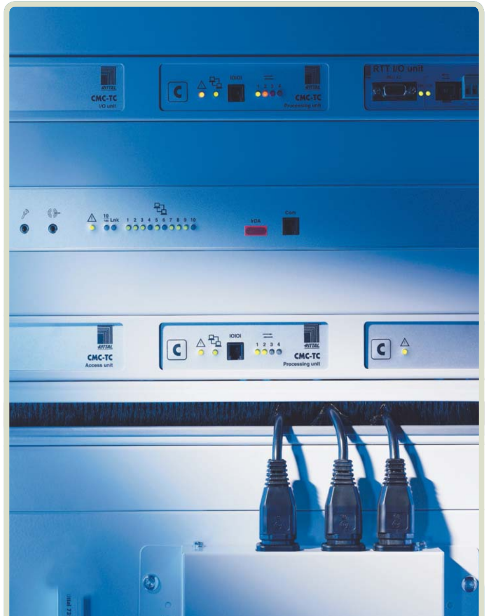
The unit has been designed to provide IT and facility managers with a centrally controlled point of information to manage physical racks and room security.
